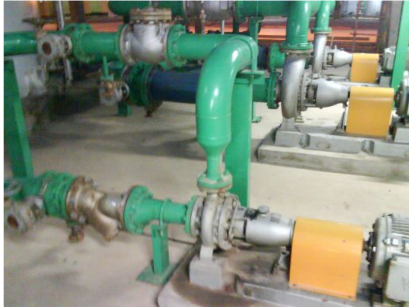
Figure 6 – Typical centrifugal pump and ancillary components installation
